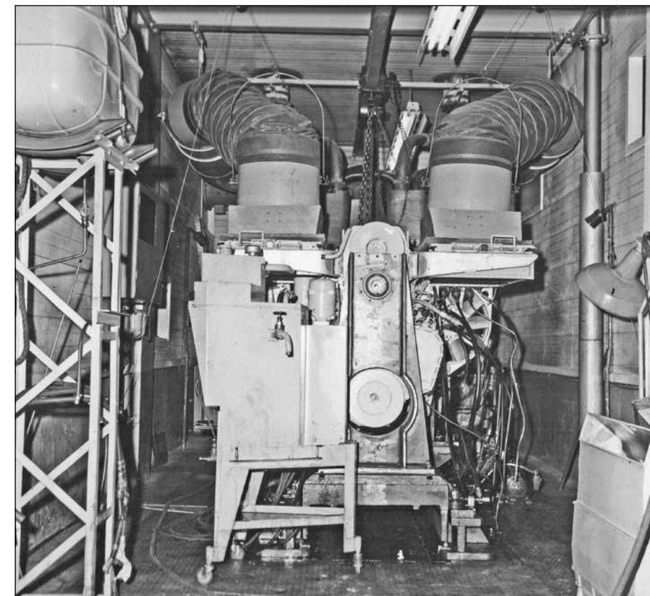
View of an L60 engine installed onto the test bed, as you can see there wasn't a lot of room! The engine was mounted on a special stand and connected to the cell exhaust and fuel system. The two large diameter pipes coming down from the roof provided air from outside the test cell for cooling purposes. The large tank on the elevated stand on the left contained a form of Lanolin (a preservative grease obtained from wool bearing animals). While the engine was running a fuel tap was switched allowing Lanolin to enter the engine, eventually the engine would run out of fuel leaving the internals coated with the preservative. These cells were used for both development and durability testing, once heard, the sound of an L60 at full throttle was not easily forgotten.
